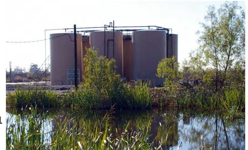
East Chalkley Tank Battery
